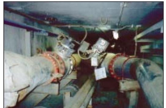
Lined Thickener Underflow Valves in Chilean Mine
