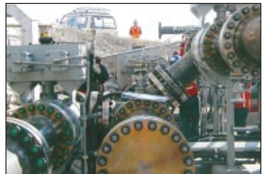
Rubber Lined Valves in Tailings Disposal System for Peruvian Mine
