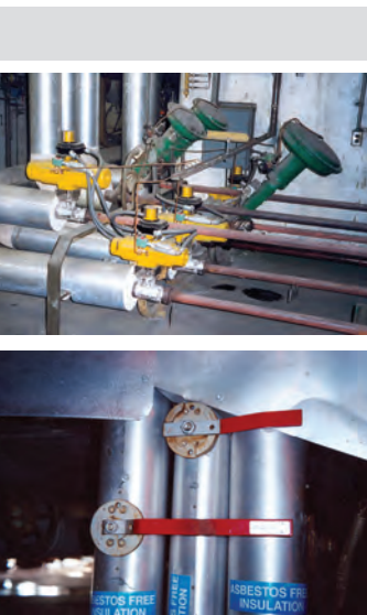
Pictured above: The function of the boiler drain and vent valves is to drain the boiler for maintenance outages. The valves are always closed when the boiler is in operation and must remain absolutely leak free while the plant is online – to ensure plant efficiency.
