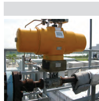
This ValvTechnologies' valve is installed in a cogeneration facility on the Gulf Coast. The application pictured is a vent valve located in the reheater section of the HRSG.
