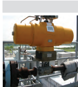
This ValvTechnologies' valve is installed in a cogeneration facility on the Gulf Coast. The application pictured is a vent valve located in the reheater section of the HRSG.
