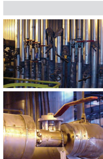
Pictured above: Main steam hot and cold reheat drain and vent valves. Steam is returned to the turbine in the hot reheat line at 1000°F (538°C), 600 psi (41 bar). The drain valves are used to heat the steam lines during start-up and discharge into condenser.
