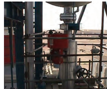
Pictured above: This Electronic Relief Valve (ERV) was installed to provide protection to the safety relief valves, which if operated could cost the plant thousands of dollars in replacement.
