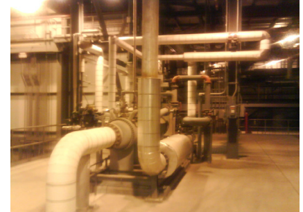
Attemperator spray block bi-directional valves operating maintenance-free for over five years
